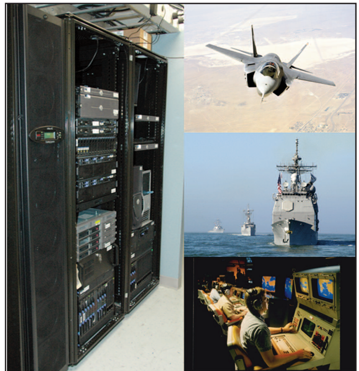
Two programs are currently underway on the Astraeus Testbed (left) in support of the both the Aegis cruiser and JSF-35 weapons systems.
